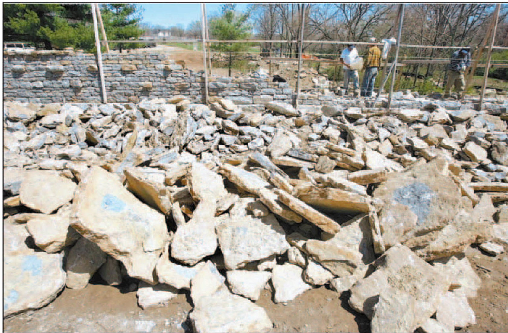
Large pieces of sandstone rock lined the road as employees with McAlister Stone fitted them together for the dry-laid stone fence.
